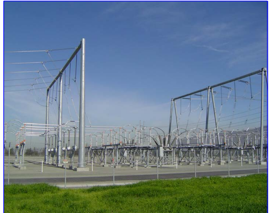
Connecting to sub at Los Esteros
